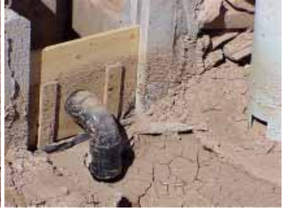
Self-Starting Siphon Installed In Drain Box
